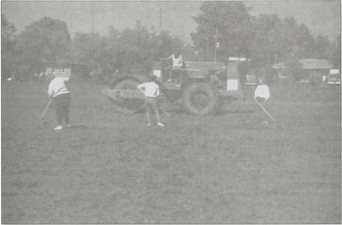
Levelling and rolling the ball diamond at the new recreation park, 1981 [Margaret Sheehey]
