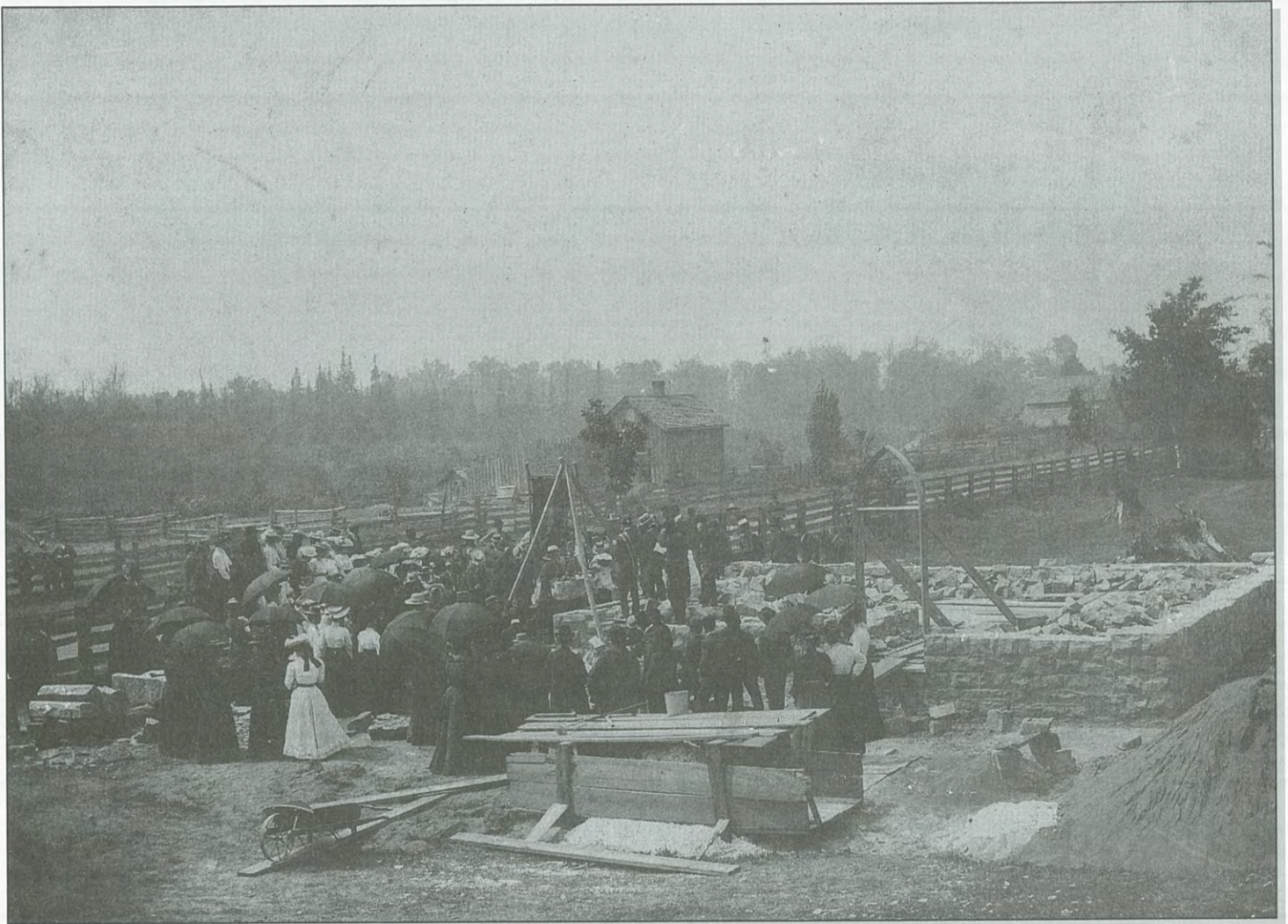
The laying of the foundation for St. Luke's Anglican Church at Burnt River in 1903 [Peggy Rettie]
